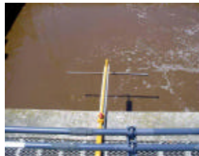
Municipality with Ferric added at the front of the aeration basin
