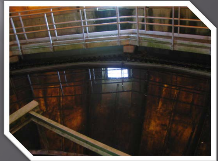
Lower levels of ashing and gassing but still scum and solids in centerwell
